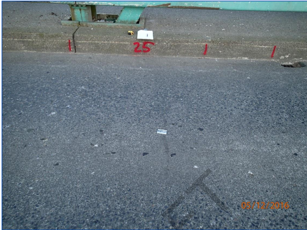
Photo 9: Partial width transverse crack near chainage 25 m in the eastbound lane.
