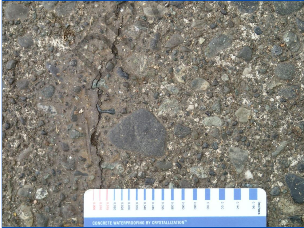
Photo 16: Close-up of Photo 15 showing 0.3 mm crack.
