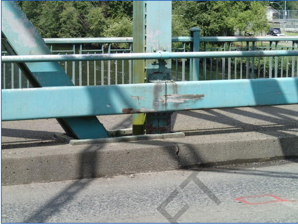
Photo 17: Minor impact damage to the north rail.
