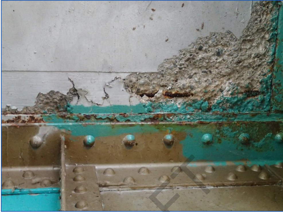
Photo 29: Spall due to low cover corroding rebar (Close-up of Photo 28).
