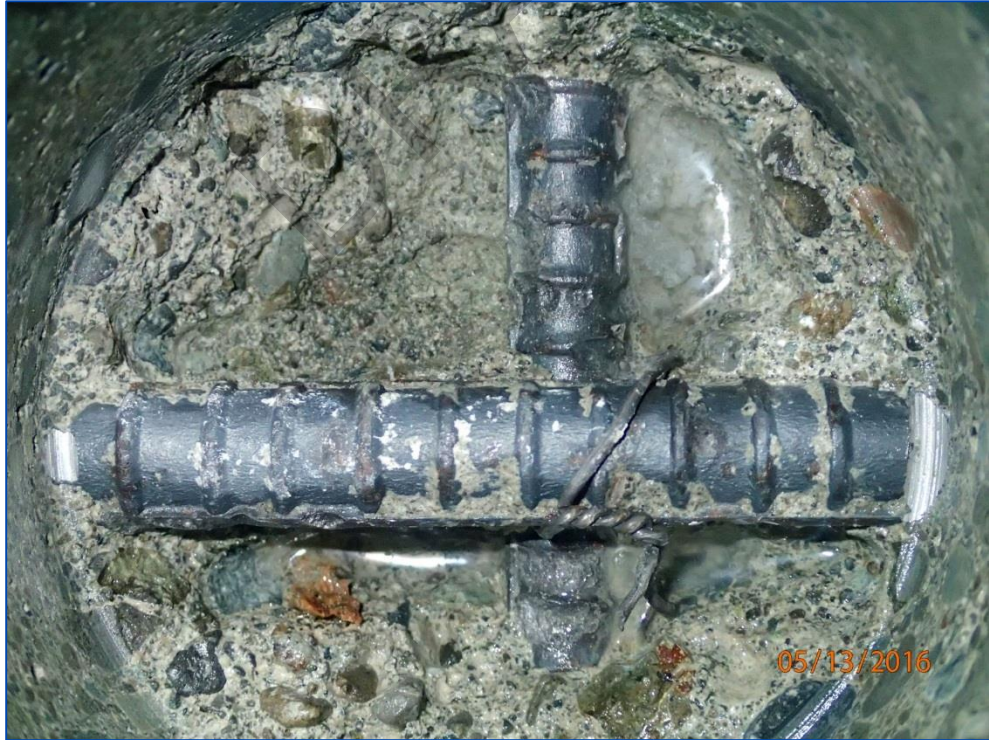
Photo 44: Condition of top mat of rebar at Core 8.
