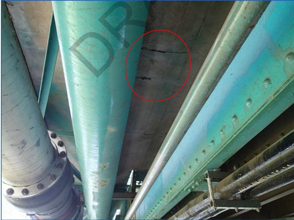
Photo 30: Spalls due to low cover corroding rebar at the north sidewalk soffit adjacent the west abutment.
