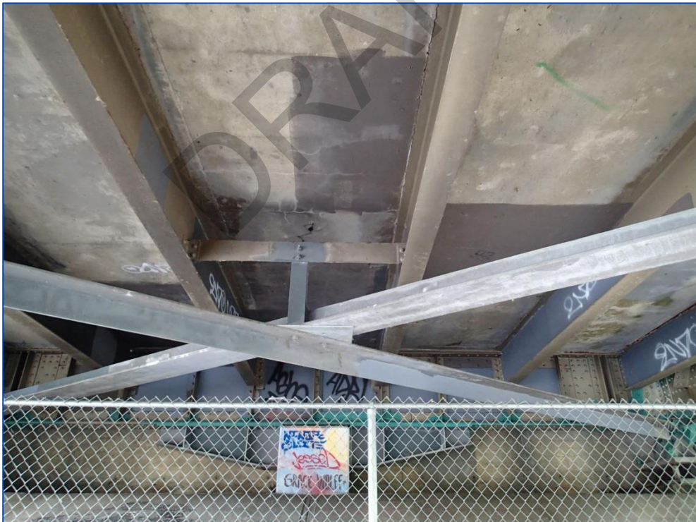
Photo 26: Soffit adjacent to the east abutment showing pattern cracking and efflorescence.
