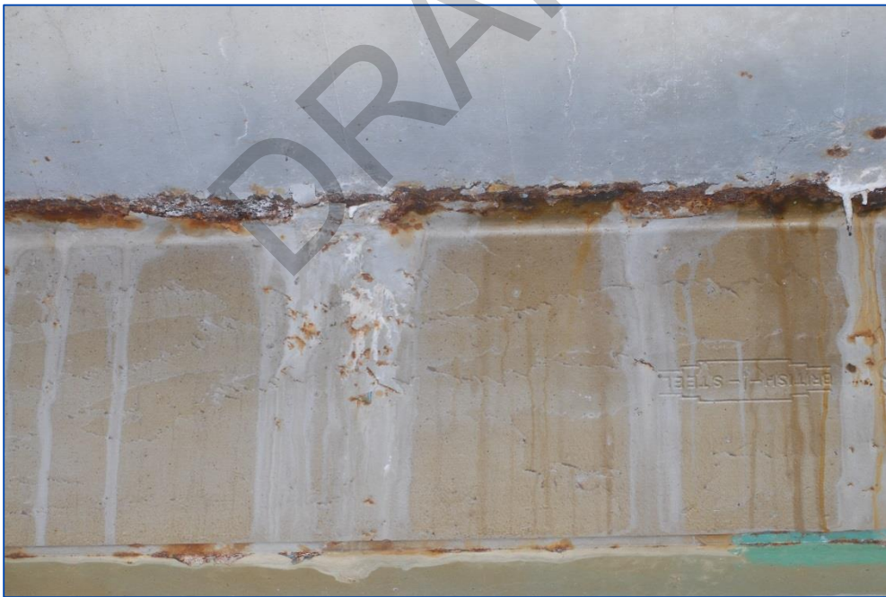
Photo 51: Close-up view of typical stringer showing corrosion of flange edge at concrete soffit.
