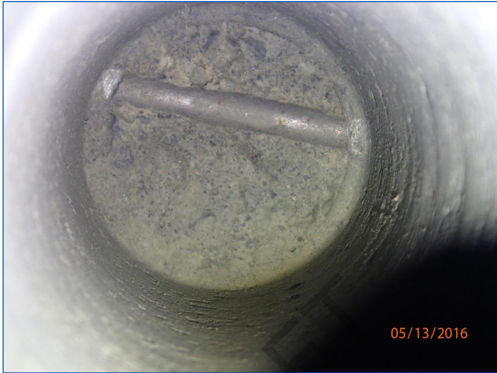
Photo 43: Condition of transverse wire mesh at Core 6.
