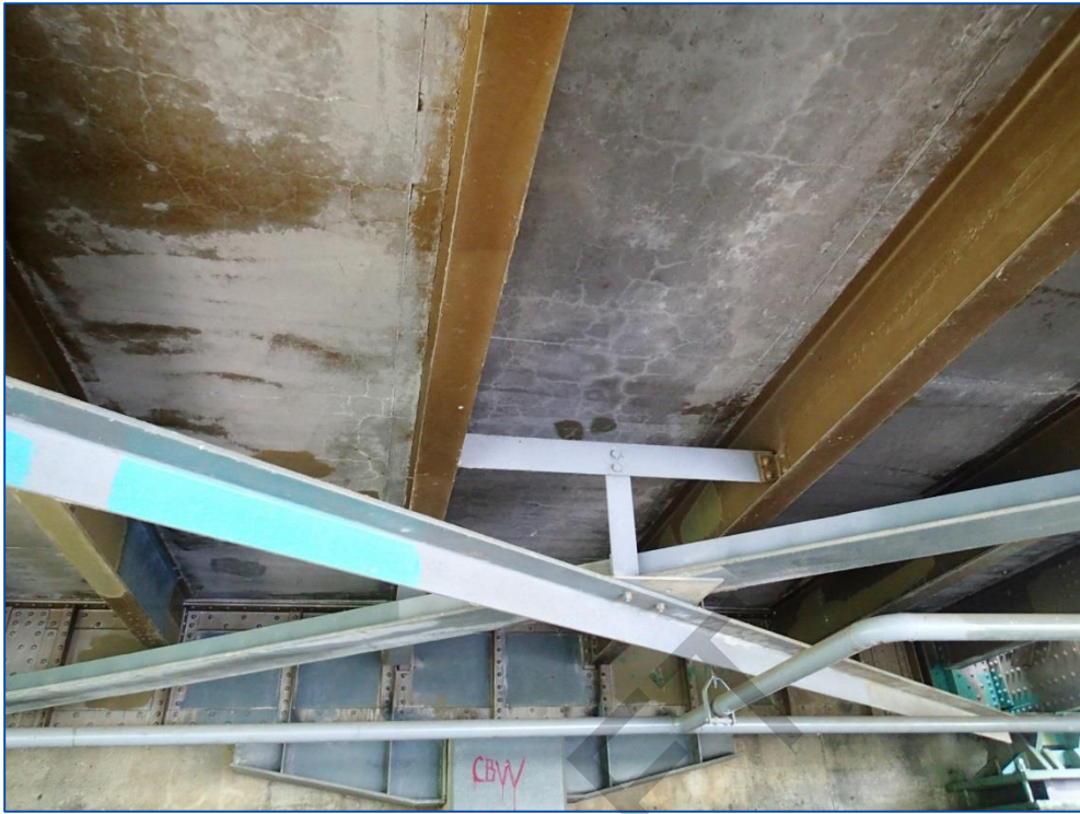
Photo 27: Soffit adjacent to the west abutment showing pattern cracking and efflorescence.
