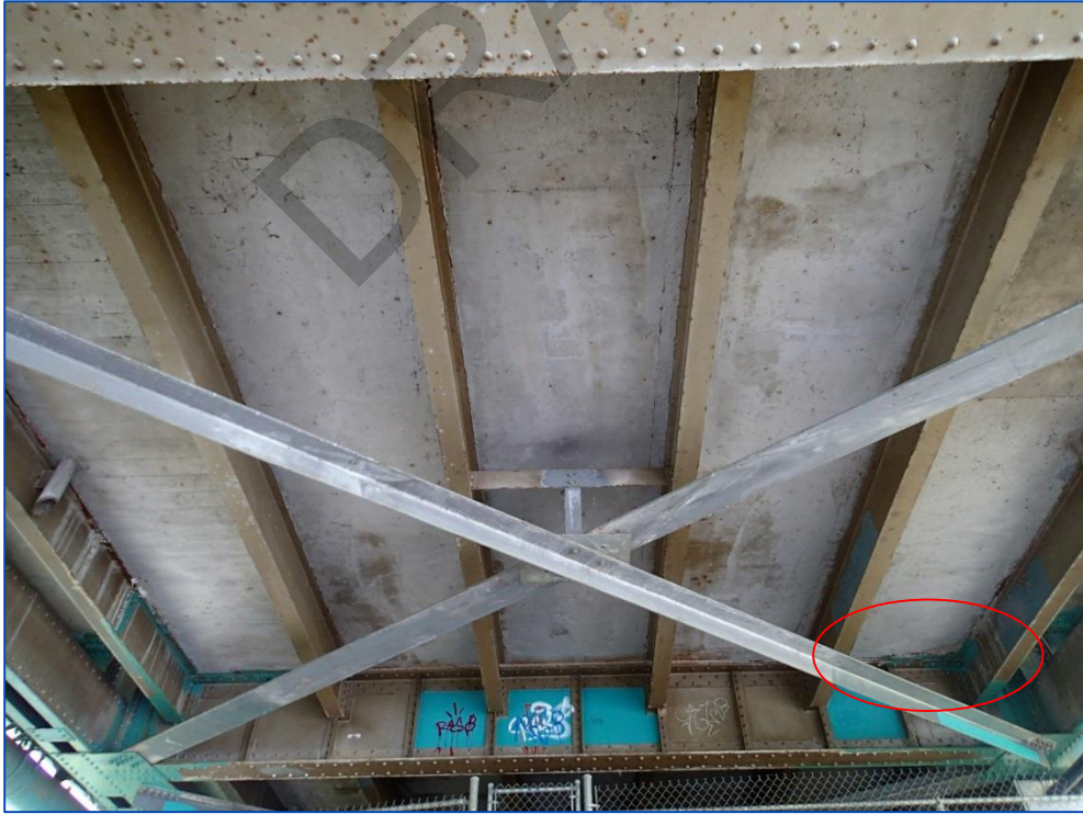
Photo 28: Soffit near the west abutment showing pattern cracking.
