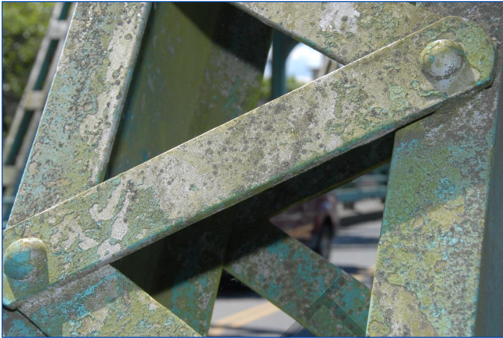
Photo 54: Close-up view of lattice in Photo 9, showing failure of green vinyl topcoat.
