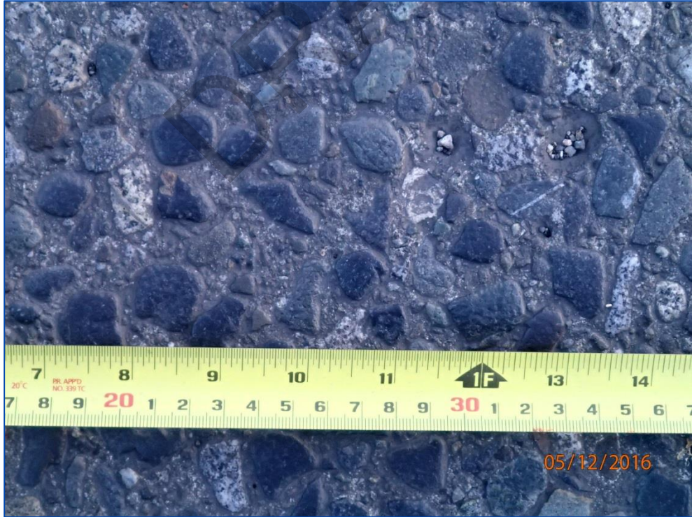
Photo 12: Moderate loss of paste resulting in exposed coarse aggregate in the wheel paths (typical).
