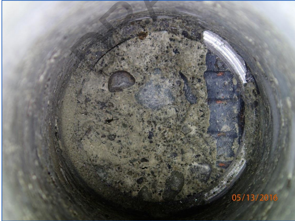
Photo 42: Condition of bottom mat longitudinal bar at Core 4.
