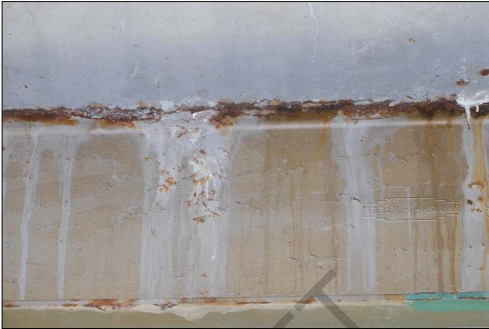
Photo 25: Close-up view of flange edge at concrete soffit.
