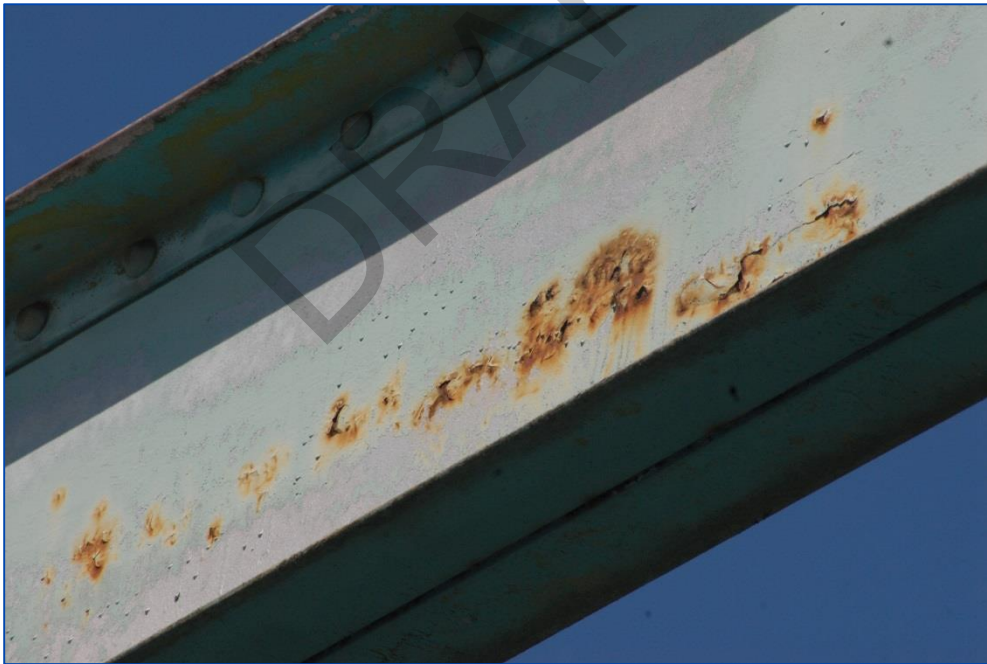
Photo 49: Close-up view of coating failure on webs of built up elements
