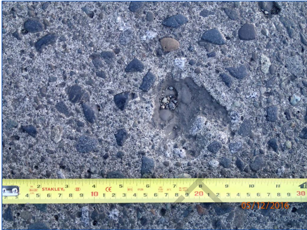
Photo 11: Minor pop out in the eastbound lane near the east end of the bridge.
