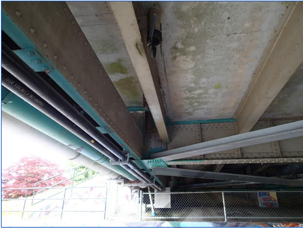
Photo 33: Northern half of deck soffit and sidewalk near the east abutment.
