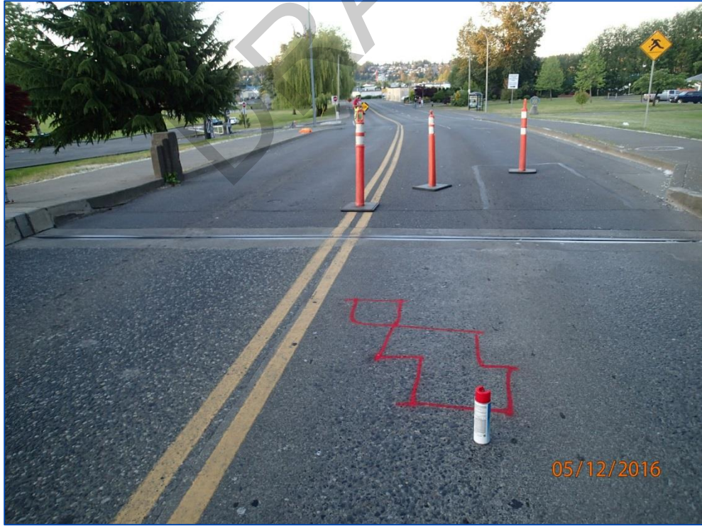
Photo 6: Delamination in eastbound lane near the east abutment.
