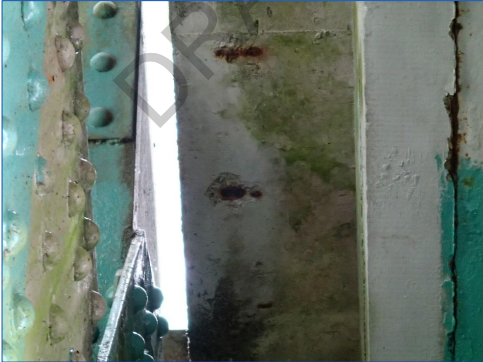
Photo 32: Low cover corroding rebar at the south curb soffit near the east abutment.
