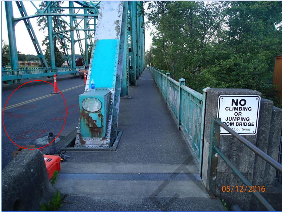
Photo 5: Delaminations in eastbound lane near the west abutment.
