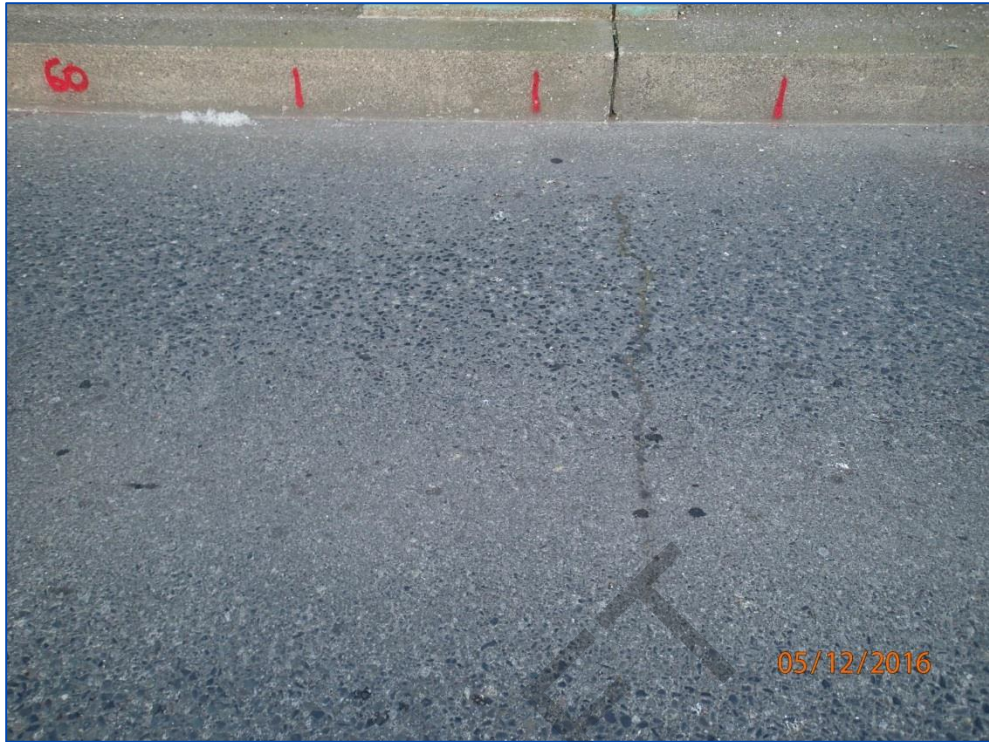
Photo 7: Transverse crack near chainage 58 m in eastbound lane.
