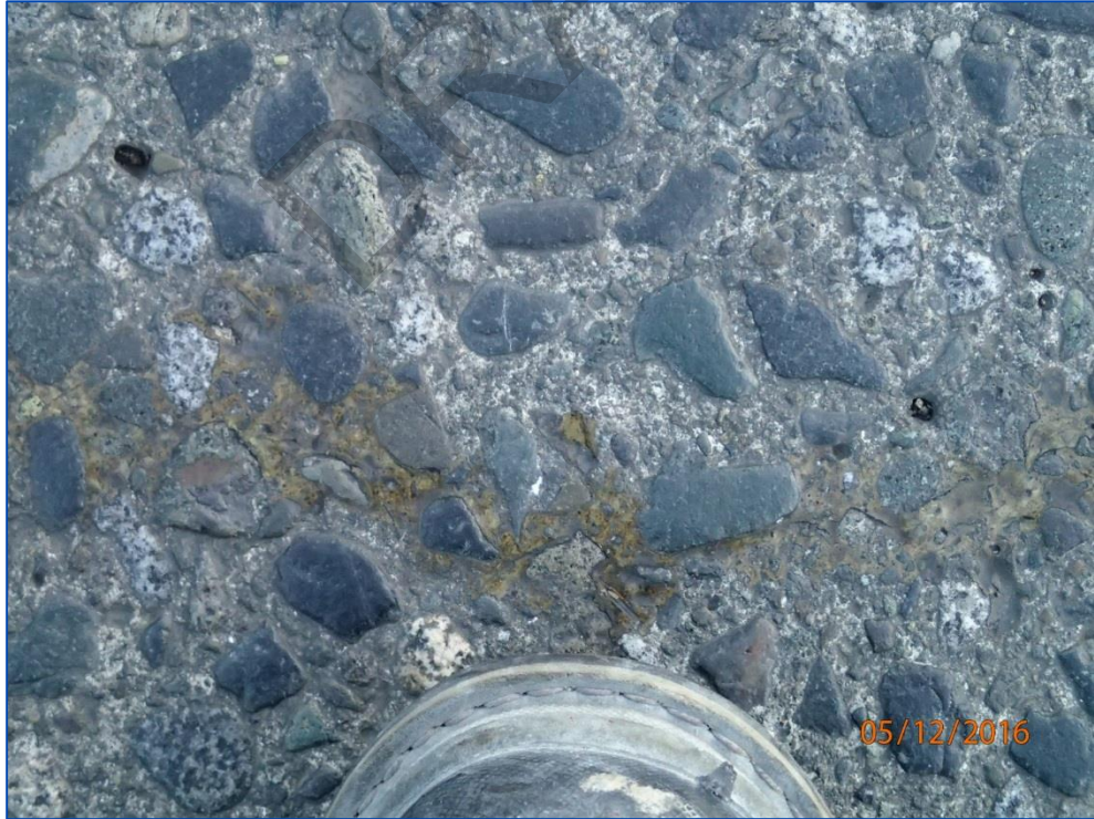
Photo 8: Close-up of a typical transverse crack in the eastbound lane with epoxy.
