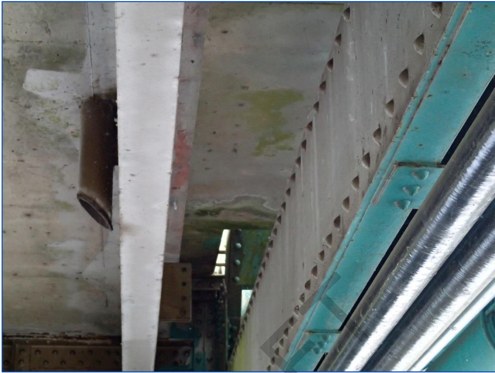
Photo 35: Leakage staining in the curb soffit adjacent to the vertical steel members (typical).
