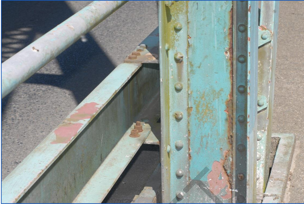
Photo 50: General view of truss "hanger" at approximately mid-span on the west (upstream) side. Note the corrosion at the toe of the angle.
